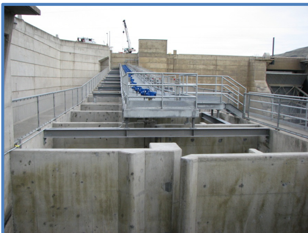
Figure 2. View of the rebuilt flow control section prior to water up for fish passage season in 2010 at the John Day Dam north ladder.
